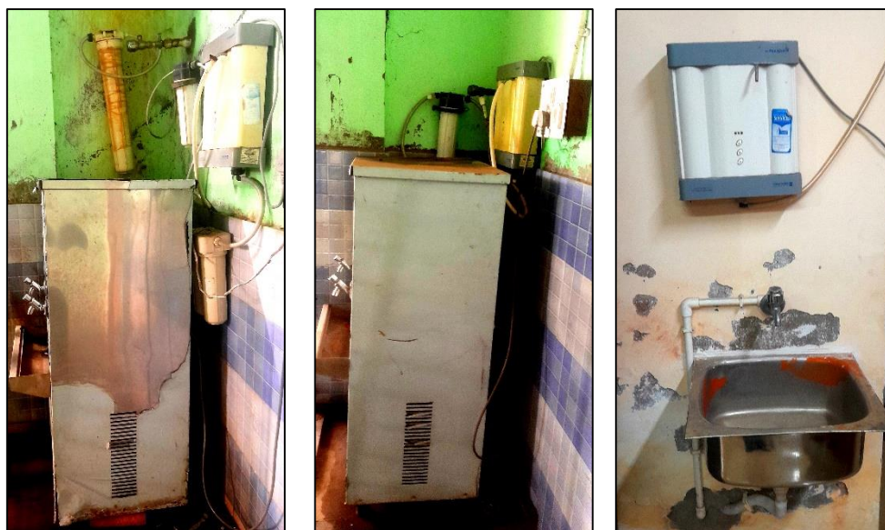
Figure 4: The filtered potable water units installed at Government General Degree College, Keshiary
